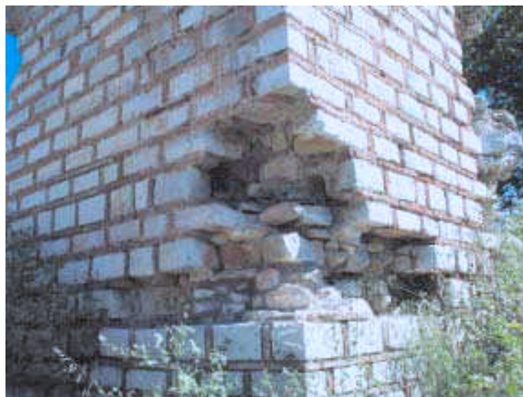
38. Vizir mosque of Nafpaktos, minaret's base, a detail of its walls' construction
