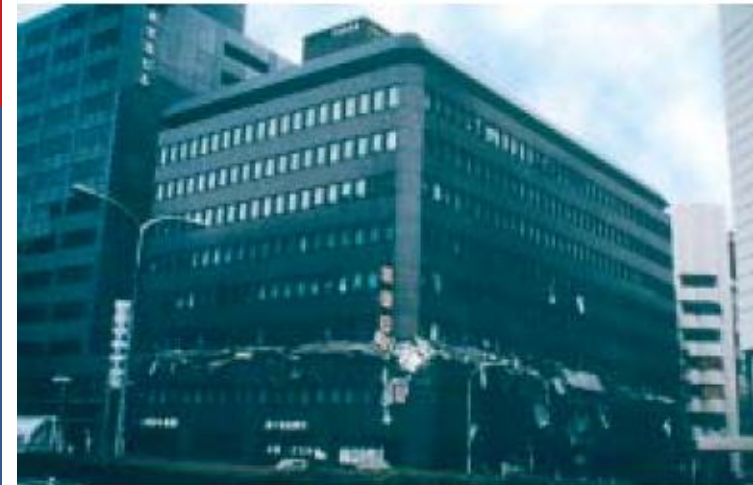
5/1 In this commercial building the third floor has disappeared and the floors above have collapsed onto it (Kobe, Japan 1995).
